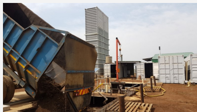
Figure 16 Loading of Feedstock Source: Renen Energy
