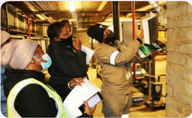
Above: The Green Scorpions inspect a refrigeration plant room in Pick n Pay-Ermelo, Mpumalanga province during a compliance intervention for users of Ozone Depleting Substances campaign.
