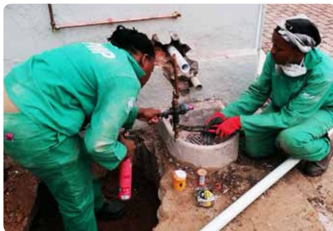
Above: Ms Thozama Gomba and Ms Lwazi Lutya installing waste water pipes for the shower.
