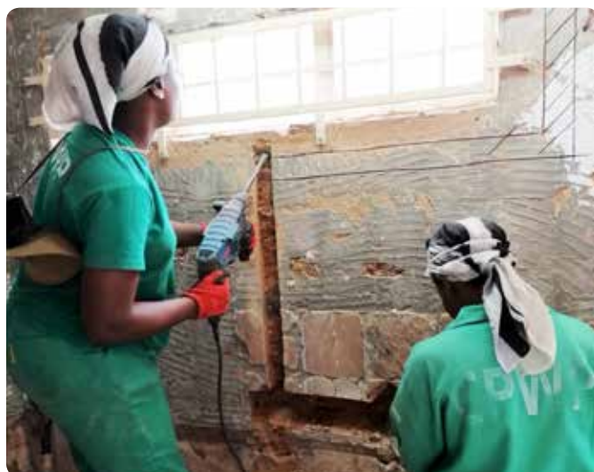
Above: Ms Thozama Gomba and Ms Lwazi Lutya of Zamava of Construction and Projects, drilling concrete wall for installation of copper pipes of hot and cold water.
