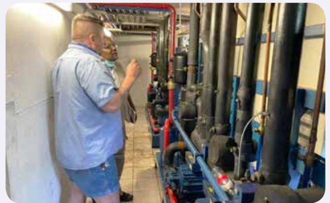
Above: Mr Larry Erasmus from JJ Erland Group demonstrates to Mr Phila Dlamini from the Chief Directorate: Sector Compliance how the pump down of the refrigeration system works.
