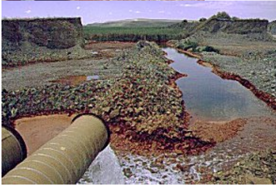
Discharge of partially treated mine water to the wetland
